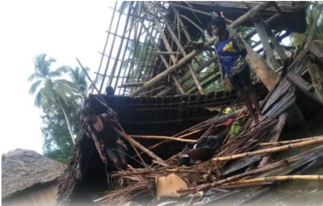
Photo House damage in the East Sepik Province.
